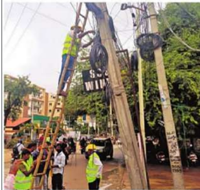
TGSPDCL employees remove unsafe cable wires from poles in Hyderabad
